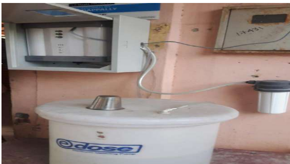
Photograph showing water purifier being installed at Govt. Higher Secondary School, Elamakkara.
